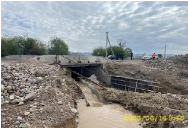
Photo 94. Lot 2. Mukandyn-Suus River bridge, km. 68+040. There are no protective measures to prevent soil from entering the river during construction works.
