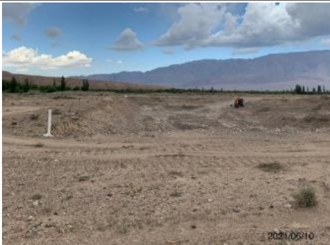
Photo 31: Quarry at km 7+100 on RHS, the quarry boundaries are marked by installing white posts.
