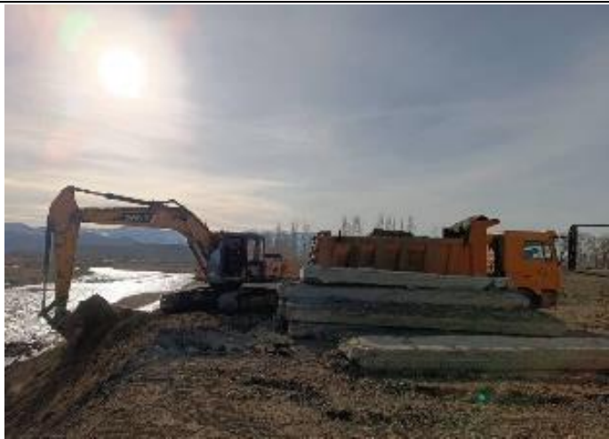
Photo 90. Dismantling of temporary bridge for bypass road at km 62+500 over Joon-Aryk River.
