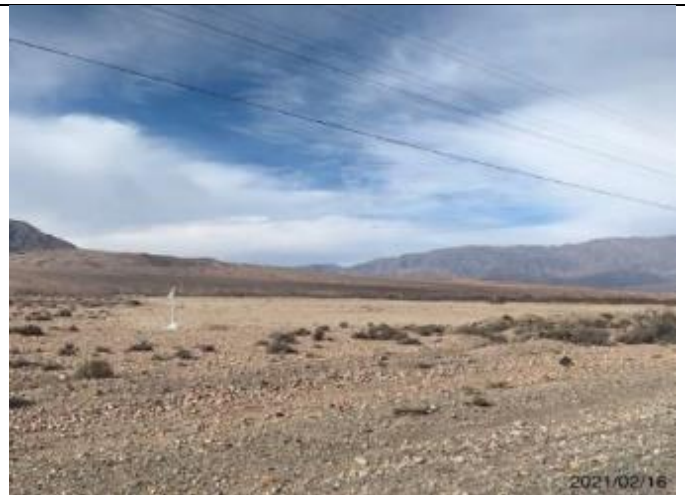
Photo 32. Lot 1. The topsoil was removed from quarry site at km.9+000, the quarry boundaries were marked by installing white posts with flags
