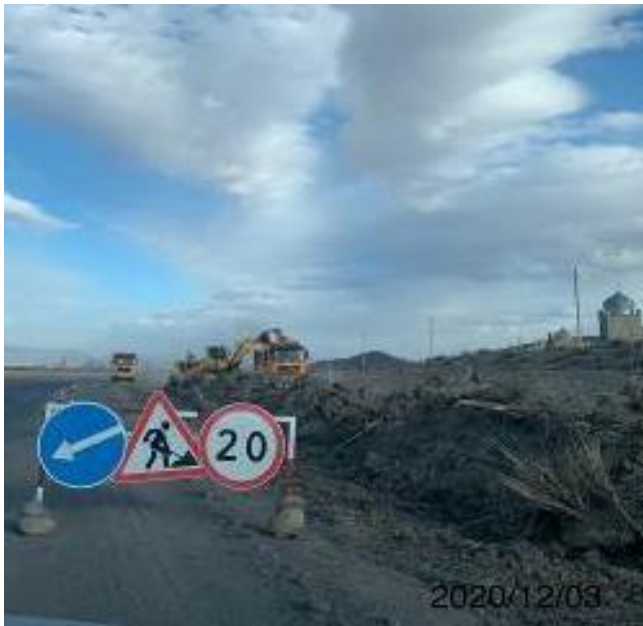
Photo 13. Lot 2. Removal of soil and vegetation layer from roadside on section km. 83+600 - km. 85+000.
