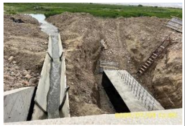
Photo 95. Lot 2. Mukandyn-Suus river bridge, km. 68+040 Water diversion is provided to prevent soil from entering the river during construction works.
