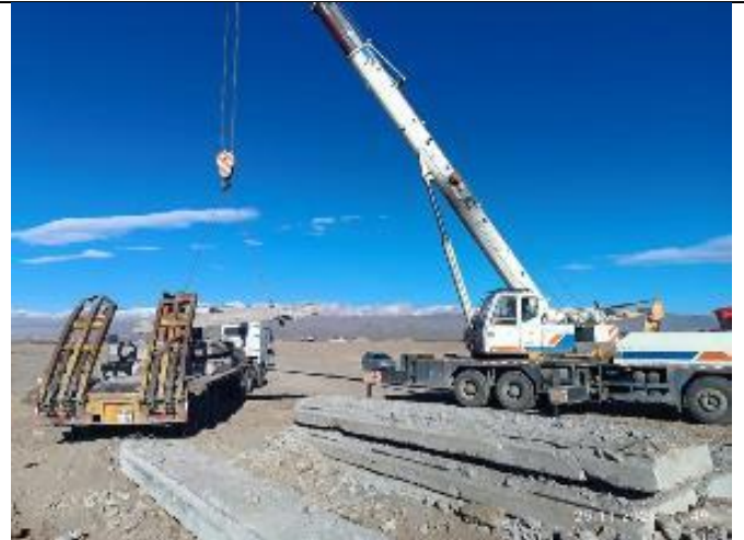
Photo 91. Removal of dismantled parts of temporary bridge for bypass road at km 62+500.
