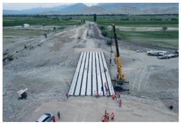
Photo 93. Lot 2. Photo 6. Construction of a bridge over the Joon-Aryk River at km. 65+410, installation of slabs.
